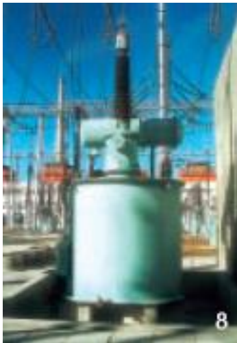
Shunt reactor (700Mvar, 154kV)
