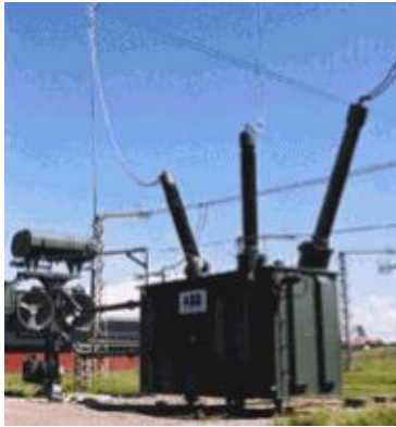
Shunt reactor (150Mvar, 400kV)
